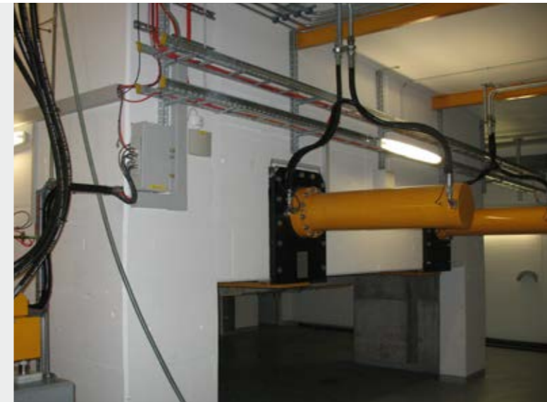
Sliding frame cylinder in a concrete silo, Sewage sludge plant Oftringen, Switzerland
