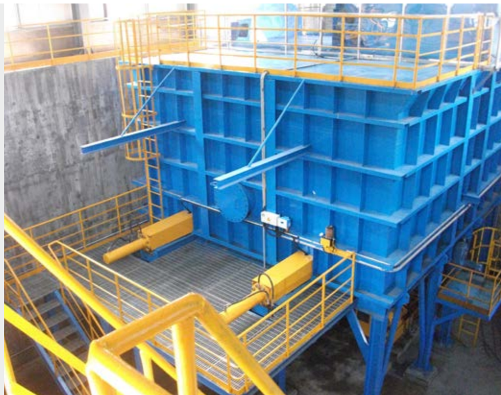
Above: Space-saving and well-proven: Drive cylinders located in the silo floor
